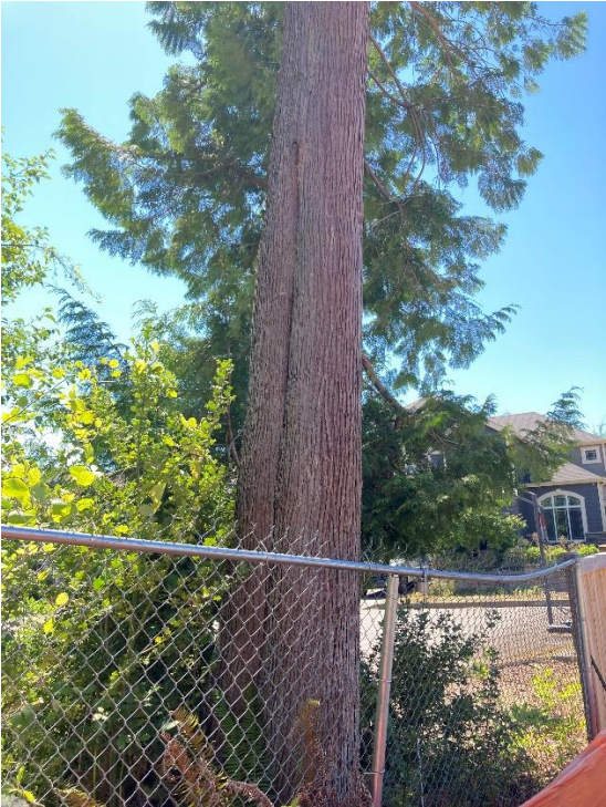
Tree No. 1 with seam and decay
